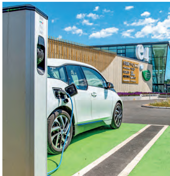
C4's electric car charging points.
