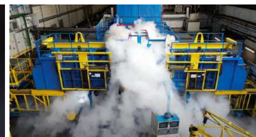
Fire protection system in Gueugnon.
